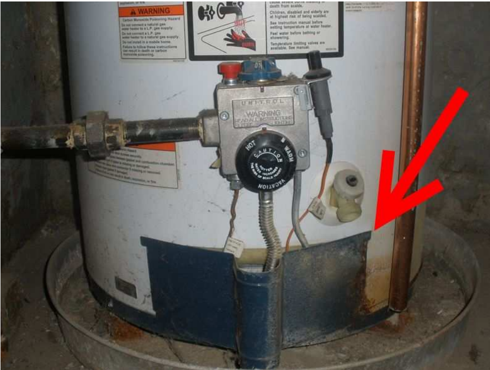
Photo # 14 water heater corrosion
